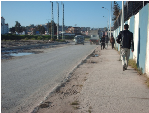
Photos 5 & 6: Sidewalks made outside standards
