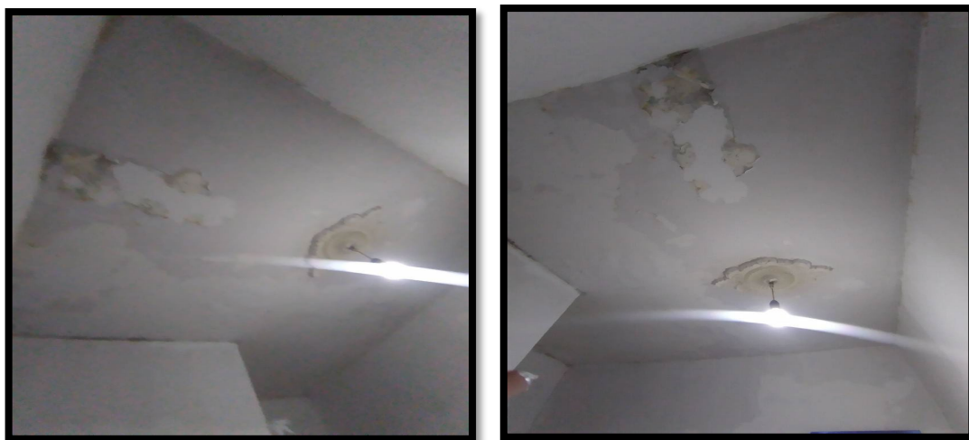
Photos N° 05 and 6: Humidity in the bathroom Source: Author 2023
