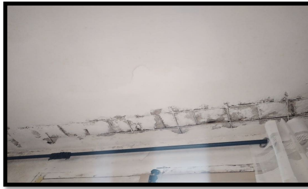
Photos N° 07: Humidity in the Kitchen Source: Author 2023
